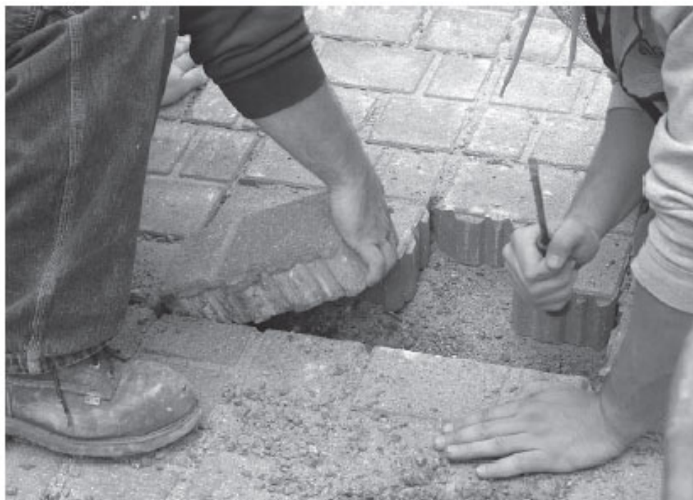
Figure 7. Pulling out a paver by the short end provides greater leverage and makes extraction easier.
