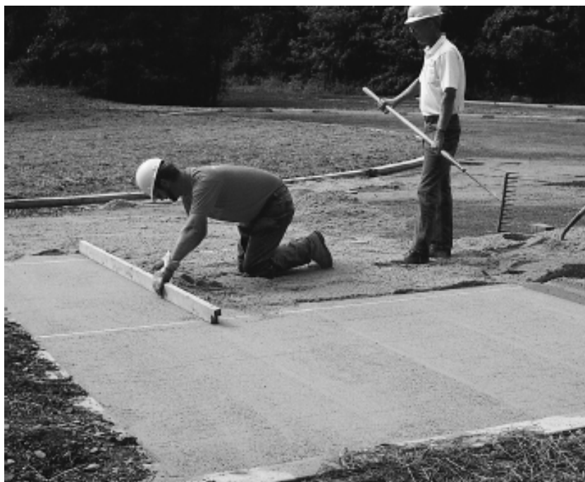
Figure 6. Screeding the bedding sand.
