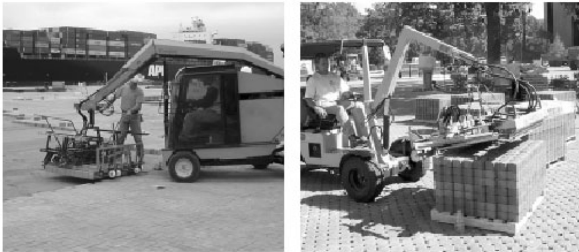
Figure 1. Mechanical installation of interlocking concrete pavements (left) and permeable units (right) is seeing increased use in industrial, port, and commercial paving projects to increase efficiency and safety.
