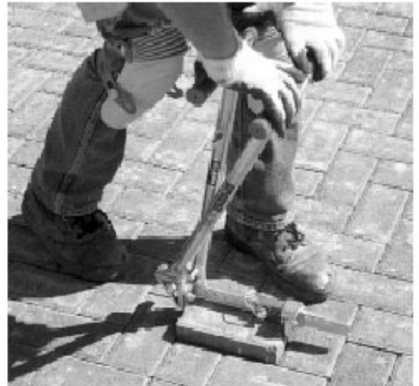
Figure 10. During initial compaction, cracked pavers are removed and immediately replaced with whole units.
