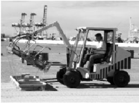
Figure 11. Sweeping jointing sand across the pavers is done after the initial compaction of the concrete pavers.
