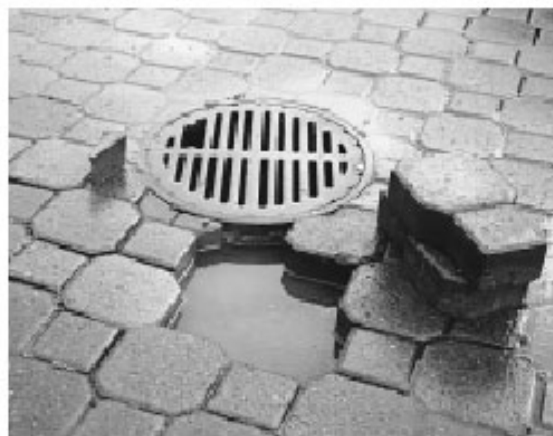
Figure 15. An absence of holes in the sides of this roof drain led to ponding.
