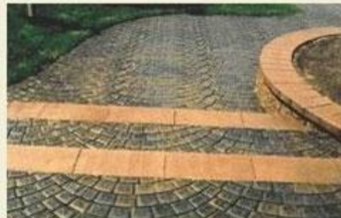
After photo of the Paving Stones after Cleaning & Sealing with STONESAVERS Surface Prep and Paving Stone Sealer.
