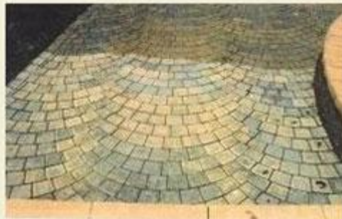
Upper part of the image is the surface cleaned to a point to show how efflorescence can obscure the true colors making paving stones look faded.
